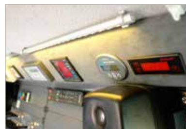
Measuring devices above side rack
